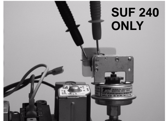
Low gas pressure switch
